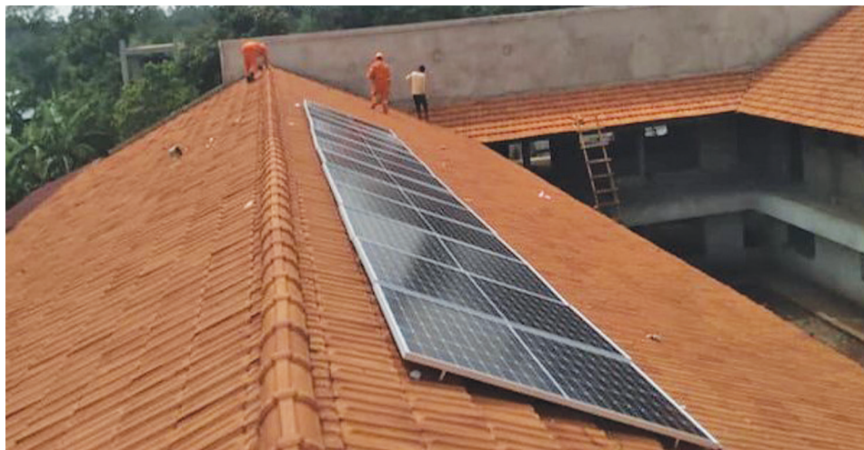
Fixing solar panels on the roof of Tororo Eco-Education and Healing Center.
